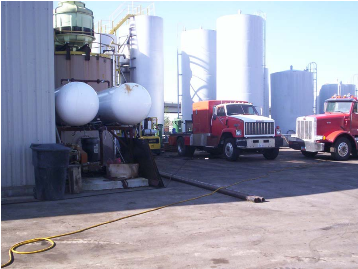
Indian Oil AST to the right and processing facility to the left
