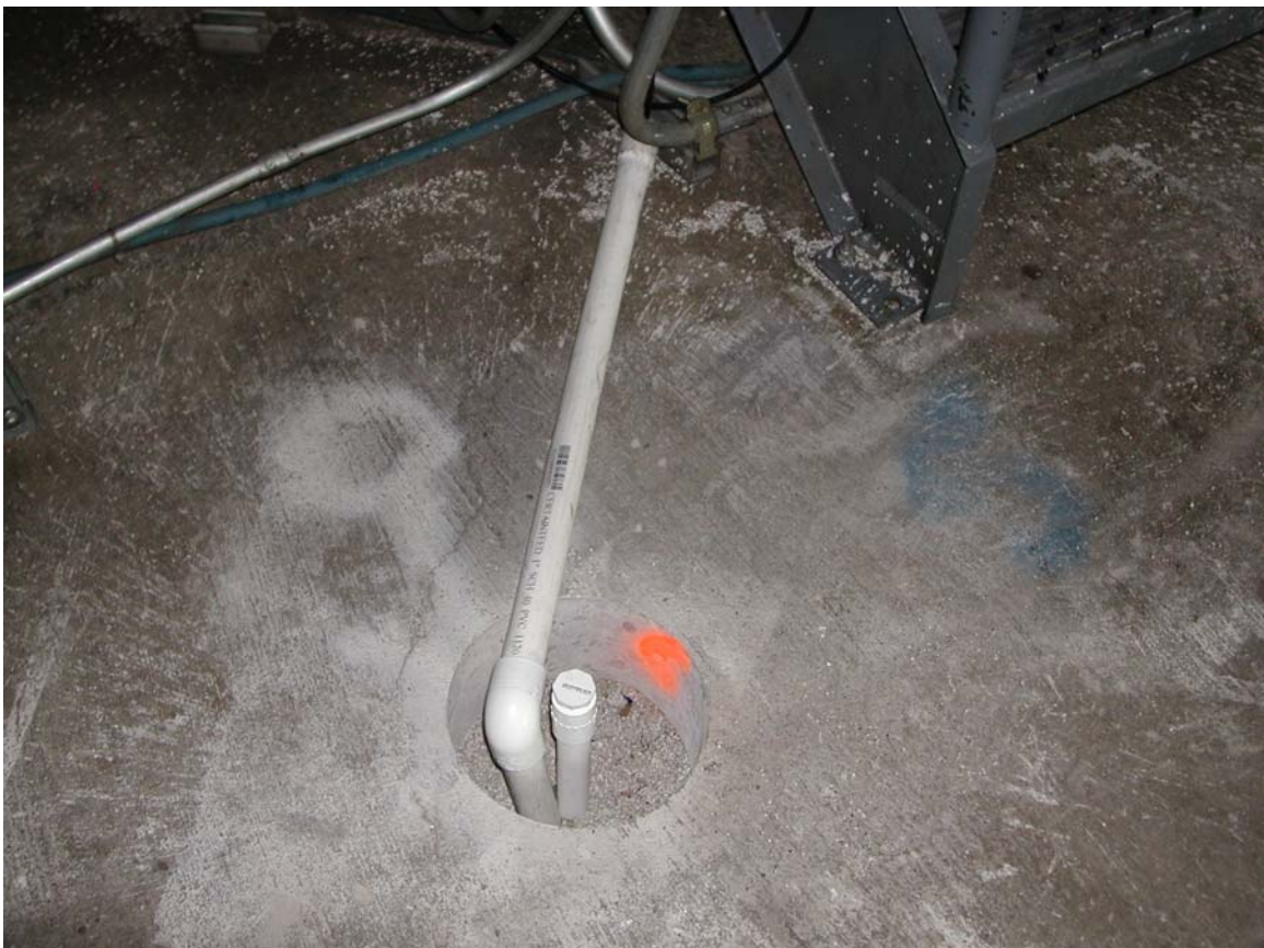
Biosparge well and nutrient well cluster in floor near stair
