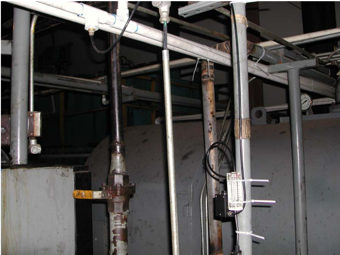
SME piping runs with facility piping; note flow controller and meter tied to pipes
